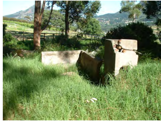
Derelict masonry water intake
