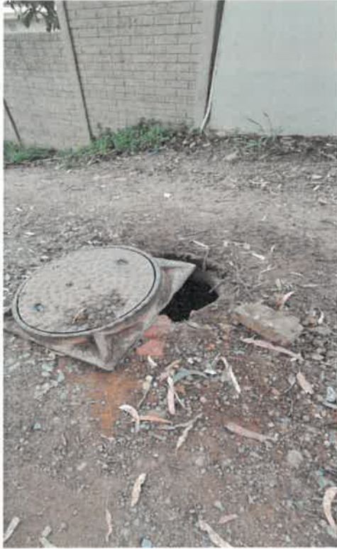
Figure 3: Photograph depicting how close this road runs to my property, no verge at all. It also shows the condition of the proposed construction access route and exposed man hole, taken in September 2024
