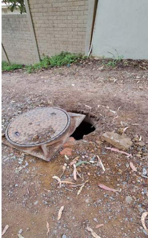
Figure 3: Photograph depicting condition of the proposed construction access route and exposed man hole, taken in September 2024
