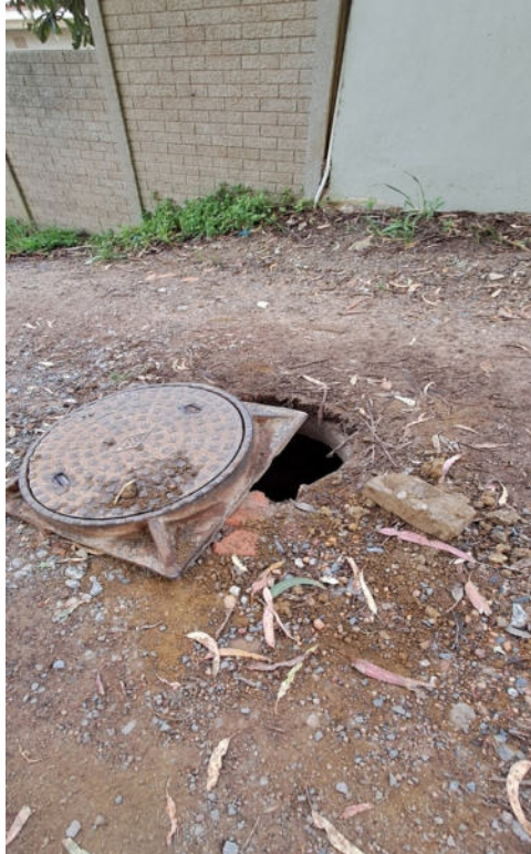
Figure 3: Photograph depicting condition of the proposed construction access route and exposed man hole, taken in September 2024
