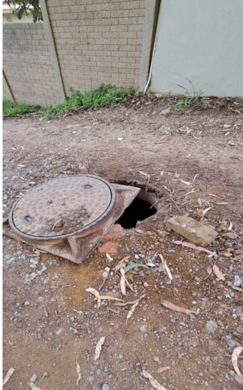
Figure 3: Photograph depicting condition of the proposed construction access route and exposed man hole, taken in September 2024
