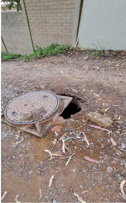
Figure 3: Photograph depicting condition of the proposed construction access route and exposed man hole, taken in September 2024
