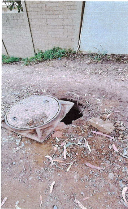
Figure 3: Photograph depicting condition of the proposed construction access route and exposed man hole, taken in September 2024
