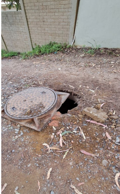
Figure 3: Photograph depicting condition of the proposed construction access route and exposed man hole, taken in September 2024
