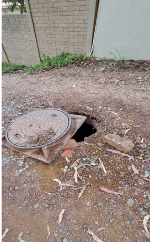
Figure 3: Photograph depicting condition of the proposed construction access route and exposed man hole, taken in September 2024
