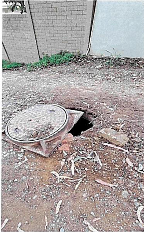
Figure 3: Photograph depicting condition of the proposed construction access route and exposed man hole, taken in September 2024
