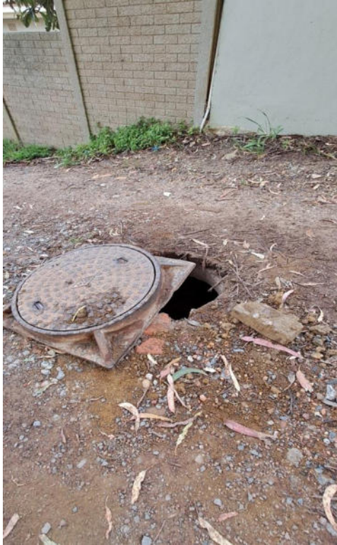
Figure 3: Photograph depicting condition of the proposed construction access route and exposed man hole, taken in September 2024
