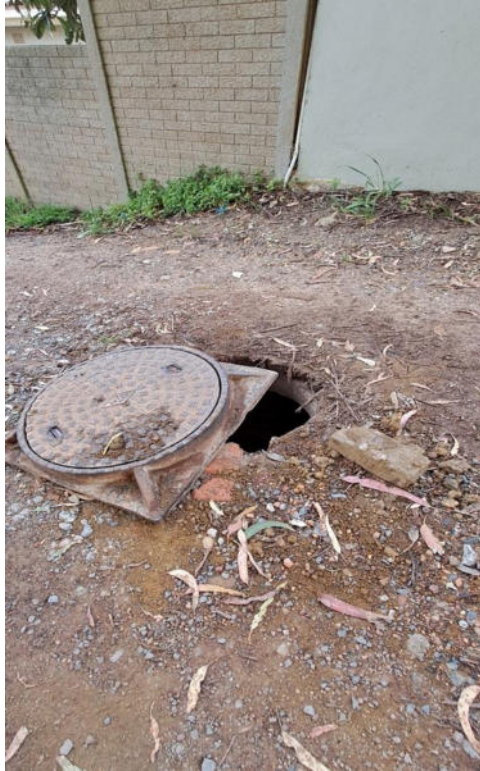
Figure 3: Photograph depicting condition of the proposed construction access route and exposed man hole, taken in September 2024
