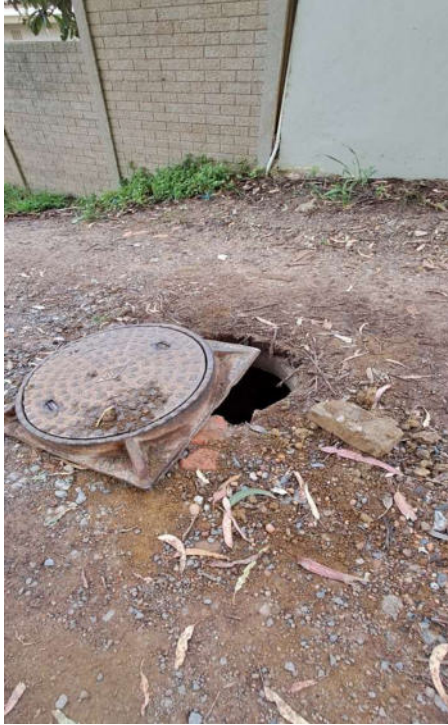
Figure 3: Photograph depicting condition of the proposed construction access route and exposed man hole, taken in September 2024
