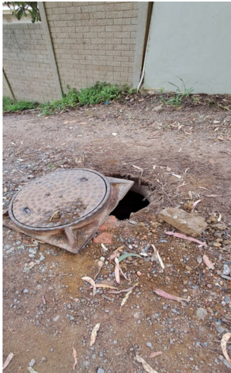
Figure 3: Photograph depicting condition of the proposed construction access route and exposed man hole, taken in September 2024
