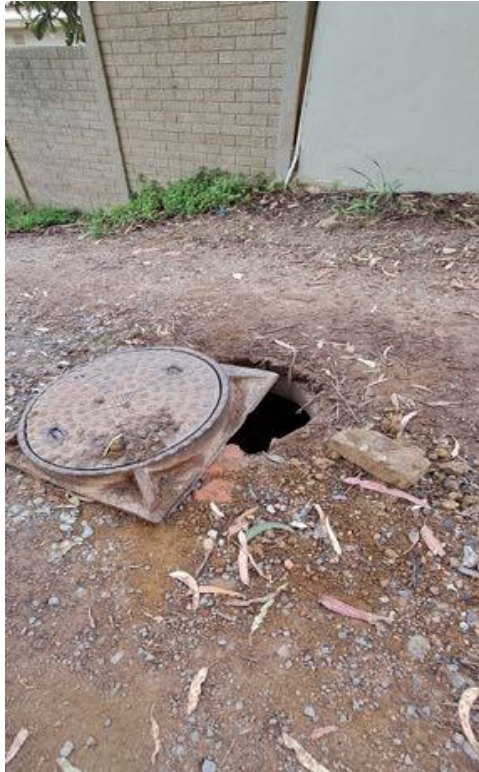
Figure 3: Photograph depicting condition of the proposed construction access route and exposed man hole on the “Old Dairy” road, taken in September 2024
