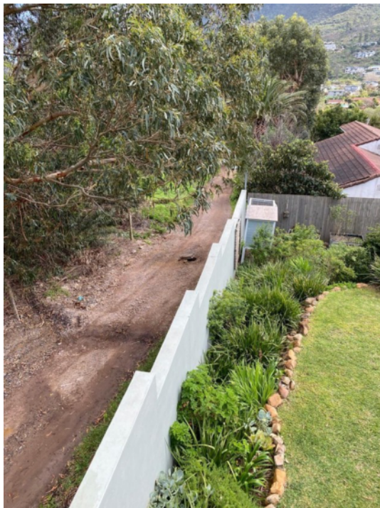
Figure 4: Photograph depicting old the proximity of the construction route and residential properties, taken in September 2024
