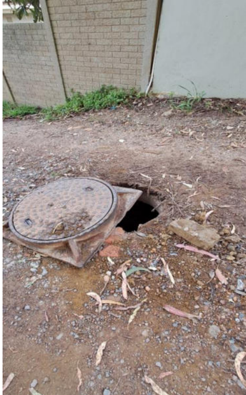
Figure 3: Photograph depicting condition of the proposed construction access route and exposed man hole, taken in September 2024
