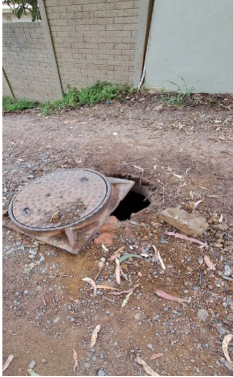
Figure 3: Photograph depicting condition of the proposed construction access route and exposed man hole, taken in September 2024
