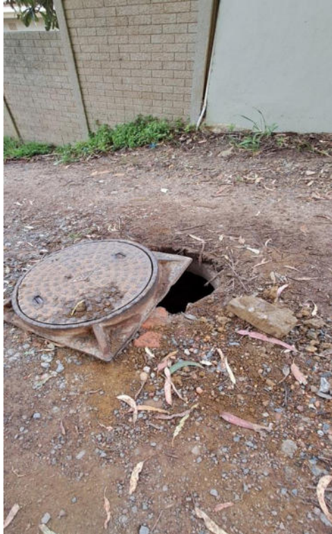
Figure 3: Photograph depicting condition of the proposed construction access route and exposed man hole, taken in September 2024
