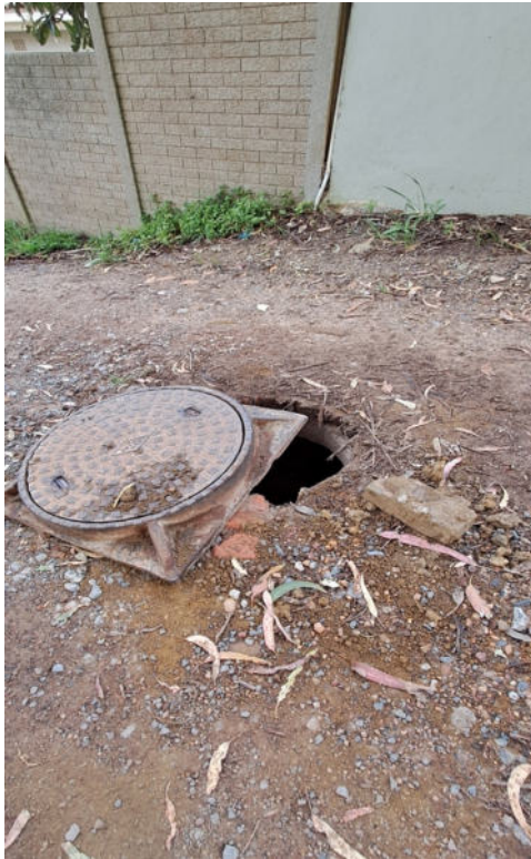
Figure 3: Photograph depicting condition of the proposed construction access route and exposed man hole, taken in September 2024
