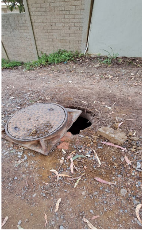
Figure 3: Photograph depicting condition of the proposed construction access route and exposed man hole, taken in September 2024
