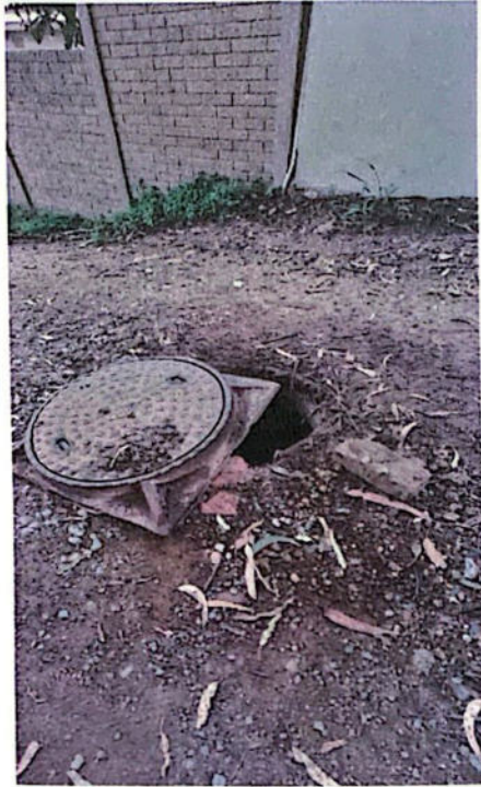
Figure 3: Photograph depicting condition of the proposed construction access route and exposed man hole, taken in September 2024
