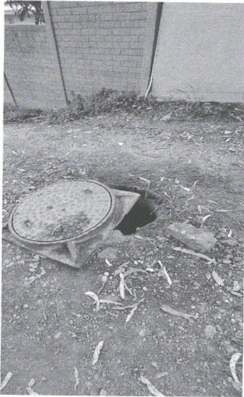
Figure 3: Photograph depicting condition of the proposed construction access route and exposed man hole, taken in September 2024
